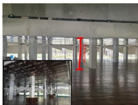
Figure 6. 114 columns in the corridor of the Baitus Shobur Mosque Source: Author's preliminary survey, 2023
